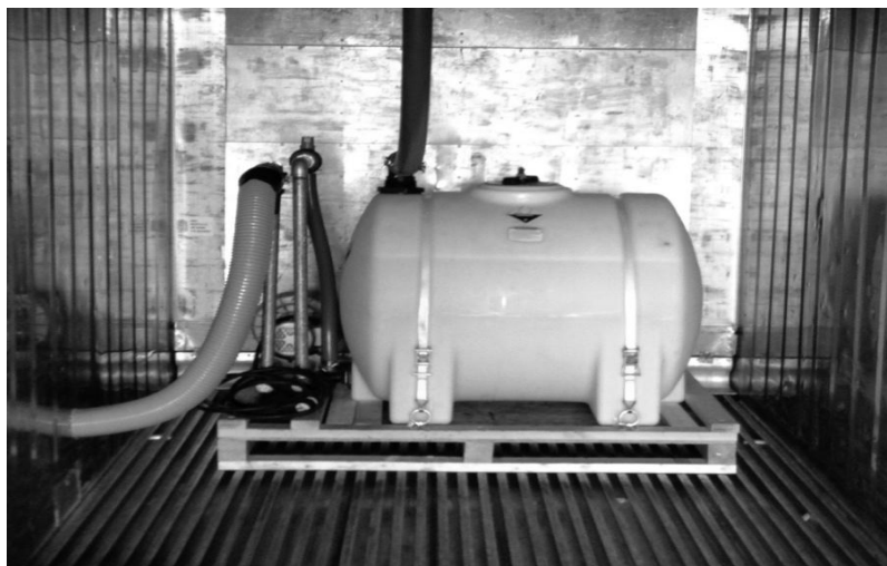
Fig. 2- Recent F.A.S.T. System Scrubber installed at Chicago O'Hare International Airport.
